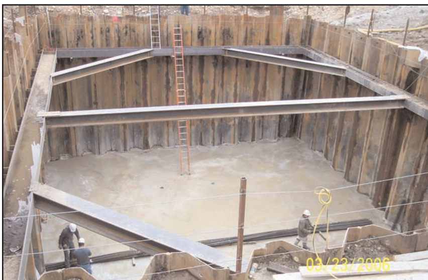
FOUNDATION work was well underway at the site of the new Main Lift Station in March 2006.
